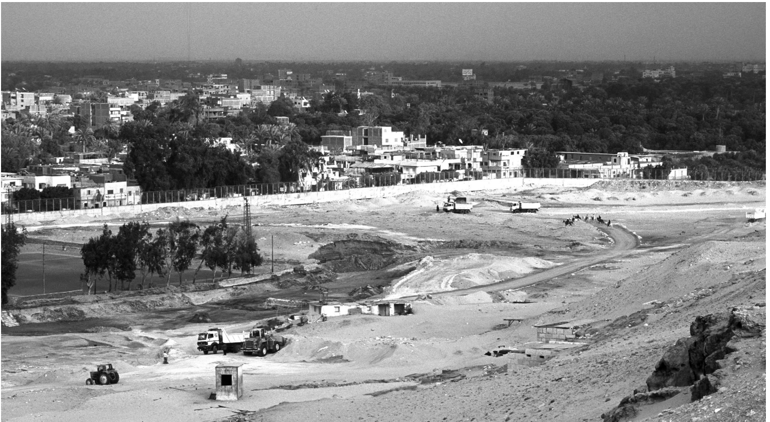
Figure 12. Clearing overburden from around the southwestern end of the Abu Hol Sports Club soccer field, which is behind the line of tamarisk trees on the left. The new access road to our site and the Workers' Cemetery can be seen on the right. The high security wall holds the town back from the archaeological zone of the low desert. View to the southeast.
